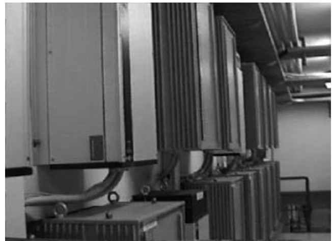
Figure 3: An array of frequency converters
